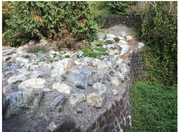
Under construction: new serpentine bog display at the Regional Parks Botanic Garden—Bart O'Brien
